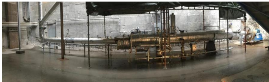
3000 hours pilot testing of Waste Heat Recovery Unit
