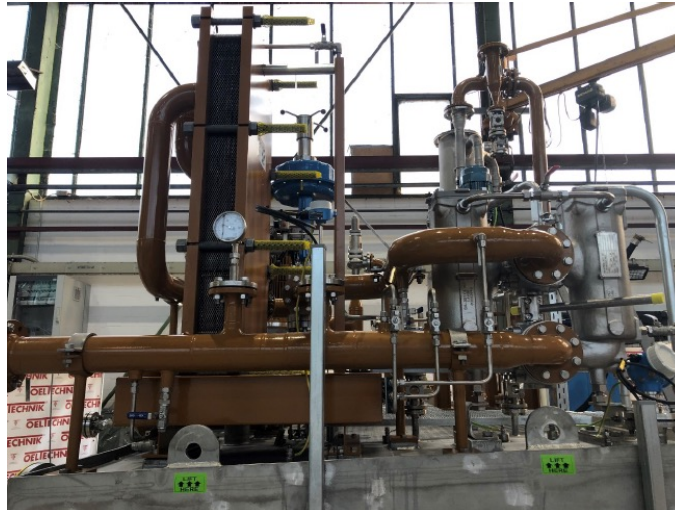
Oil lube unit
